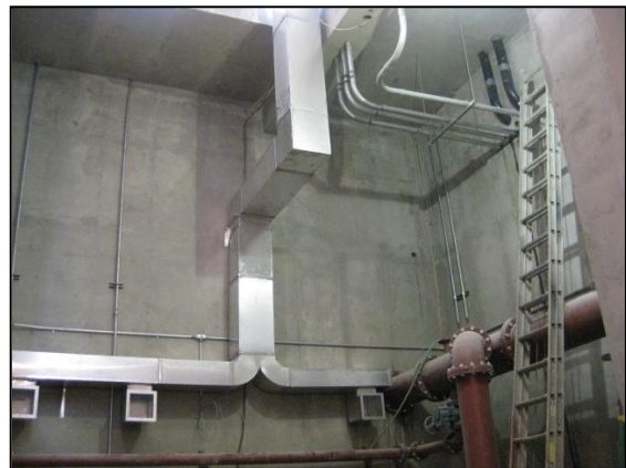
HVAC Ducting and Electrical Leading to Dry Pit – Pump Station 720
