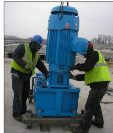
Aerator Motor for Oxidation Ditch
