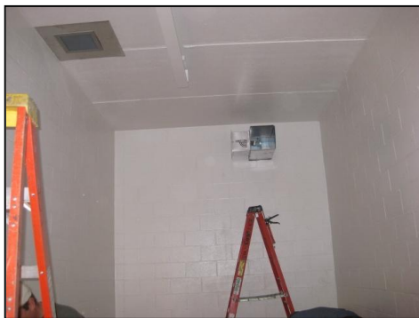
Epoxy Paint and HVAC Ducting – Pump Station 710
