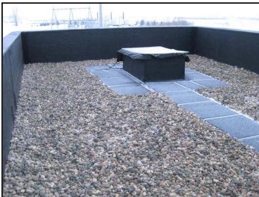
Balasted Roof System with Walkway Pads
