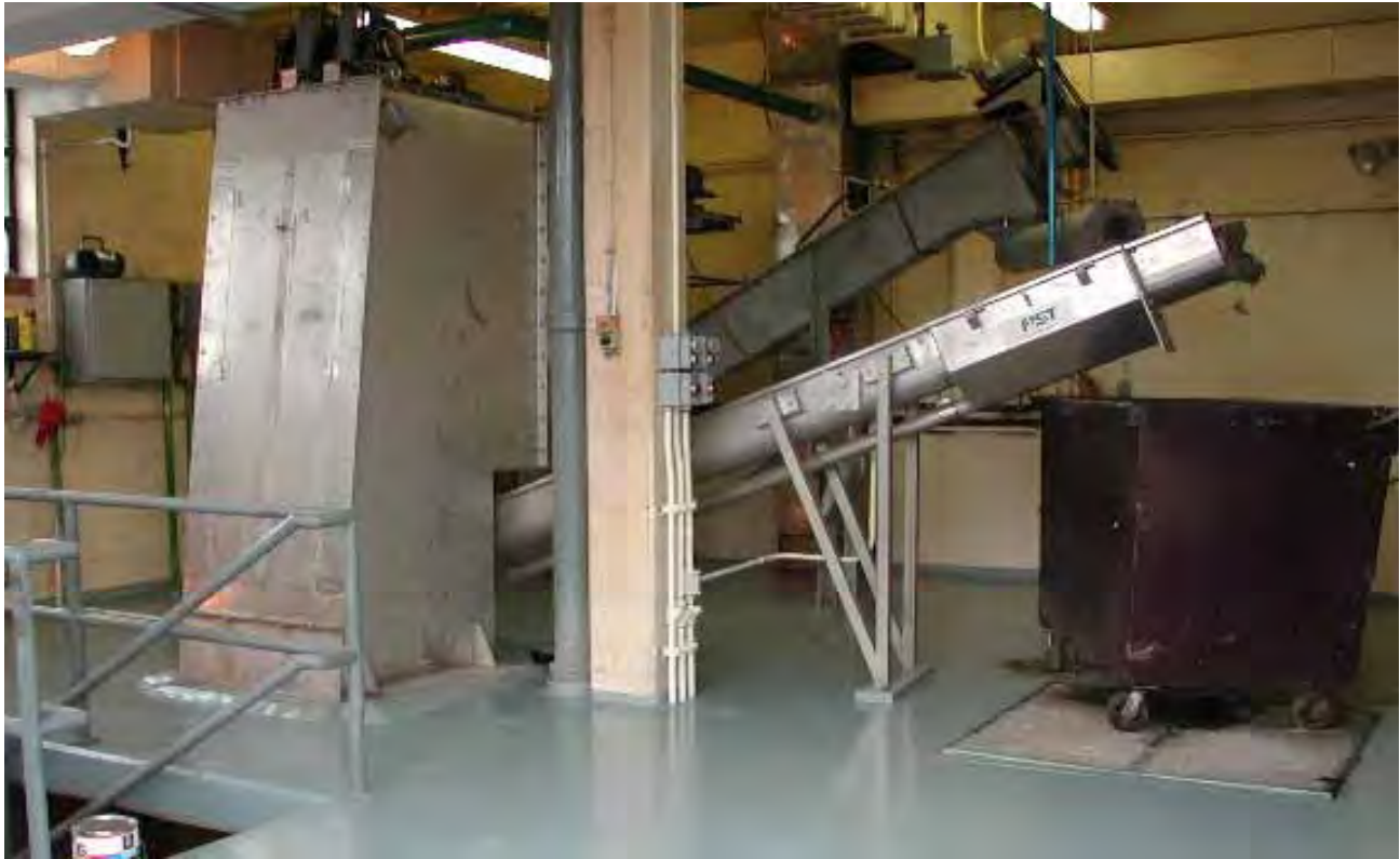
Course Barscreen and Compactor
