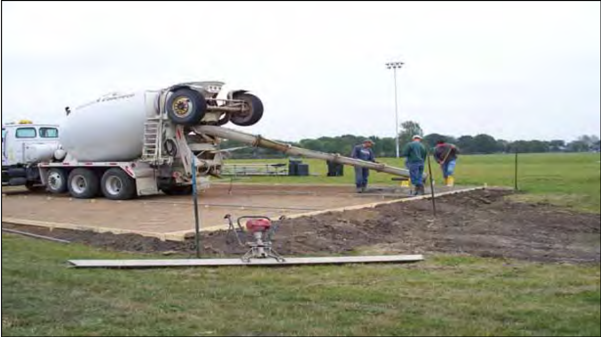
Public Works crews installing concrete bleacher pads at the Soccer fields by Roosevelt School.
