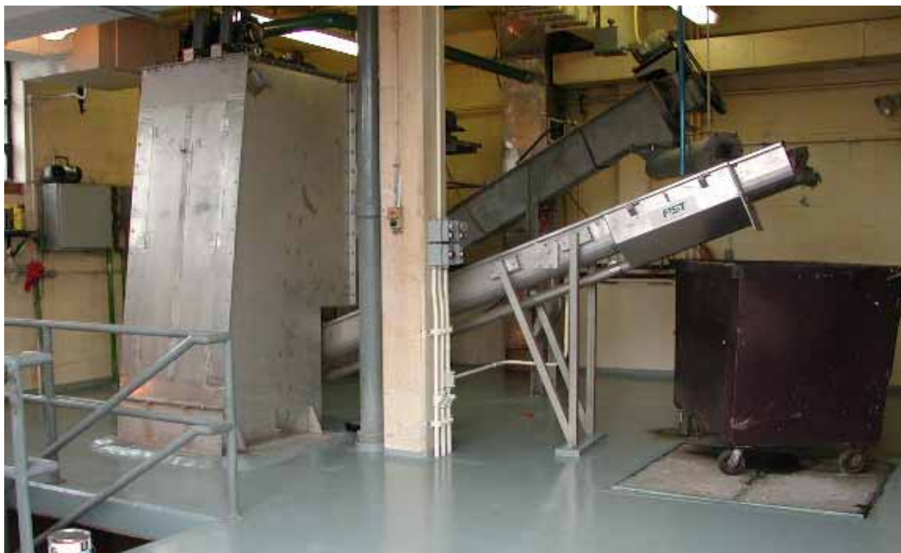
Course Barscreen and Compactor
